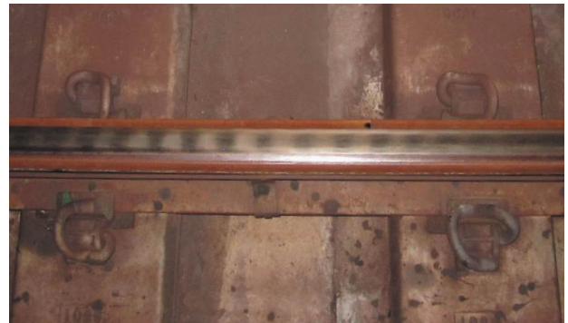
Corrugation at Adjacent Control Section
