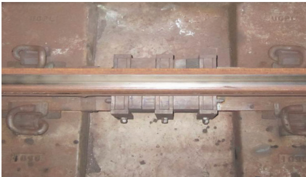
Slight Corrugation at Damper Section (E Type)
